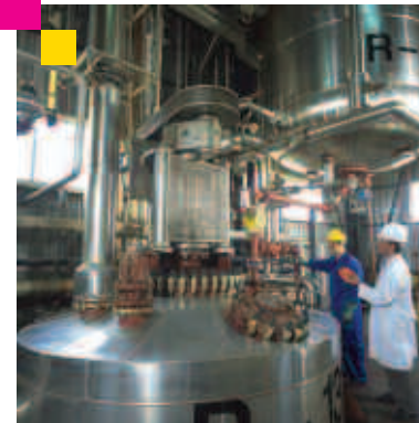
View of the reactor where the EDDHA chelating agent is synthesised. Tradecorp's production plant in Ávila (Spain)
